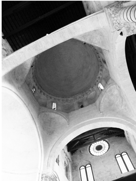
Figure 7: The Dome in the Roof Construction inside the Cathedral S. Sabino of Bari
