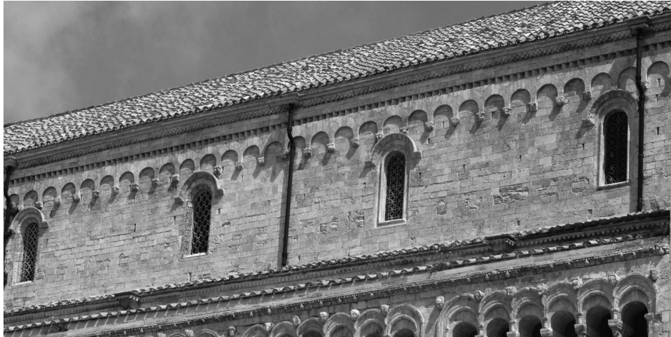
Figure 14: Stone Windows in the Central Nave of the Cathedral S. Maria Assunta (Bitonto)
